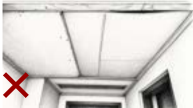
Conventional Dilapidated wooden trapdoors
